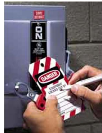
FIGURE 3 - Deactivate and mark HVAC system at electrical panel (use LOTO procedure and indicate date, time and name of person applying the tag)
