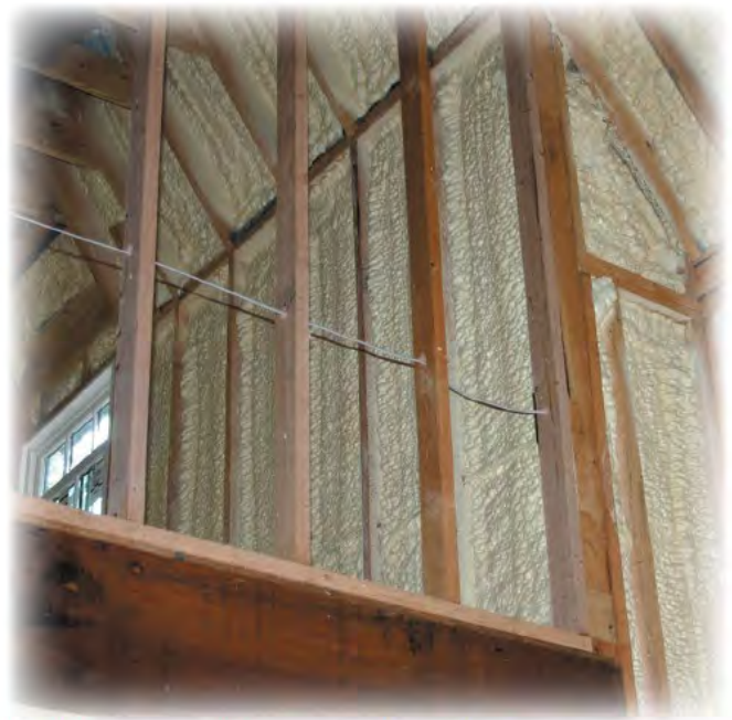
With the home well encapsulated in SPF, it was important to downsize the air conditioner. Bigger units in well-insulated homes tend to not run long enough to allow humidifiers to properly remove moisture.
