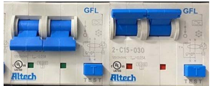
Bank 3 Breaker Open/ Tripped (OFF)
