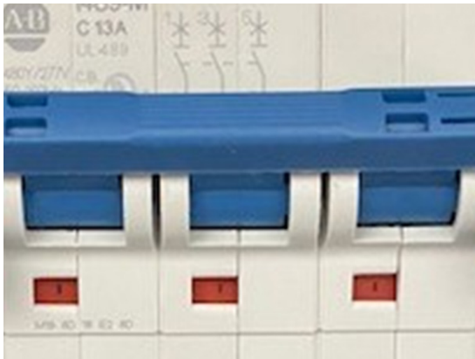
Bank 1 Breaker Closed/Hot
