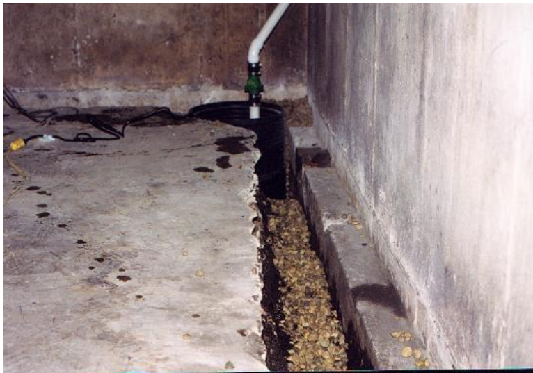
Figure 1 – Interior Foundation Drainage System with Sump Pump
