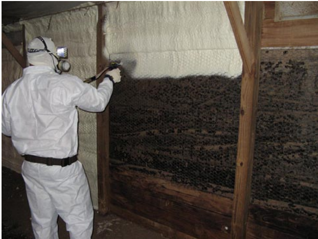
Applying spray foam to the interior sidewall with one inch of foam seals the house and changes the R value of the curtain to about R-8 and the R value of a wood wall to about R-9. Heat loss through the wall is reduced by 75-80%.
