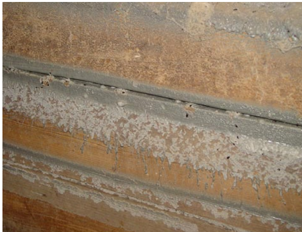
If sprayed-on polyurethane foam is to be used, protecting the cured insulation from bird pecking and beetle damage like that shown here is essential.
