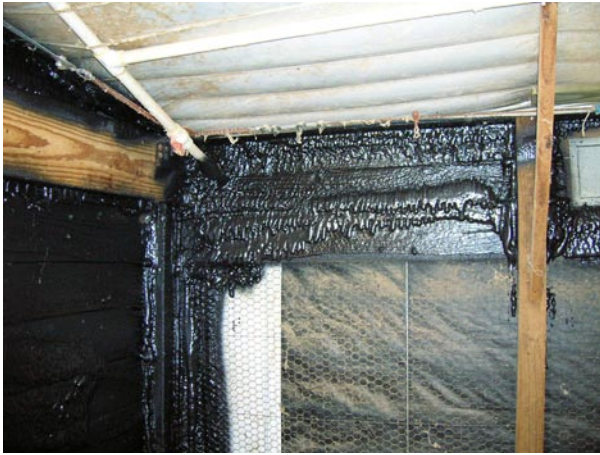
Photo shows spray-on polyurethane foam above the tunnel inlet, often a difficult area of the house to get air-tight.
